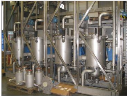
Four separators in one skid
