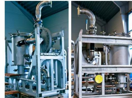
Air Oil separators front and back.
