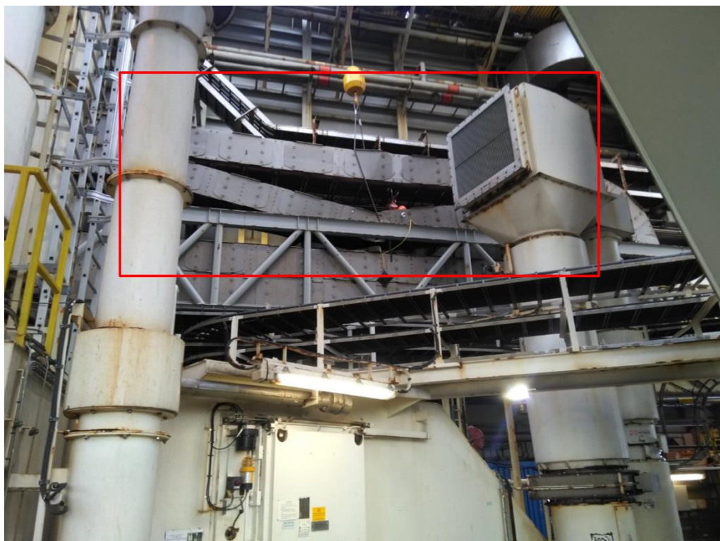
Figure 2 The collapsed drag chain and the surrounding area after the IP had been freed. Source: Odfjell Technology
