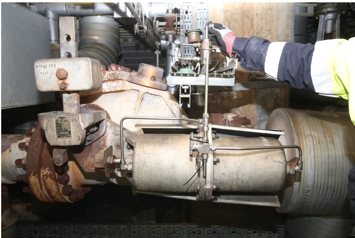
Figure 6 The Flintstone valve after the incident (source: Kripas).
