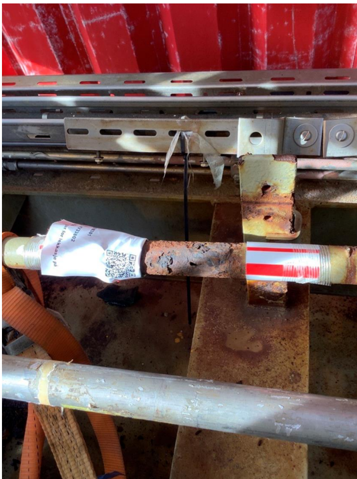
Image 4 Leak point 2, UK metering station. SFB. (Source: taken during PSA investigation)
