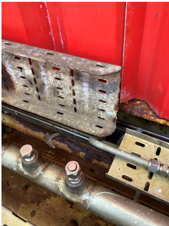
Image 2 Leak point 1, Statpipe metering station. SFB. (Source: taken during PSA investigation)
