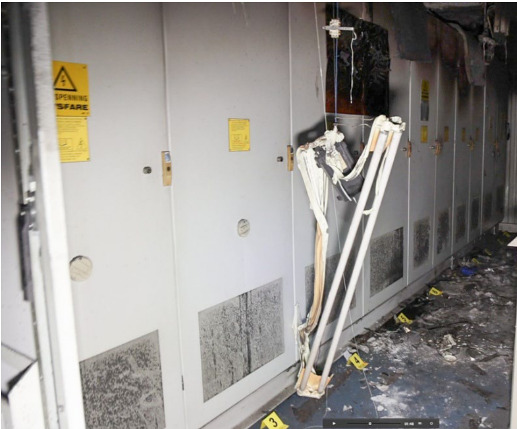
Figure 10 Photograph of the VSD after the fire. The photograph shows cabinet doors 2 to 11. (Source: Norwegian Police)
