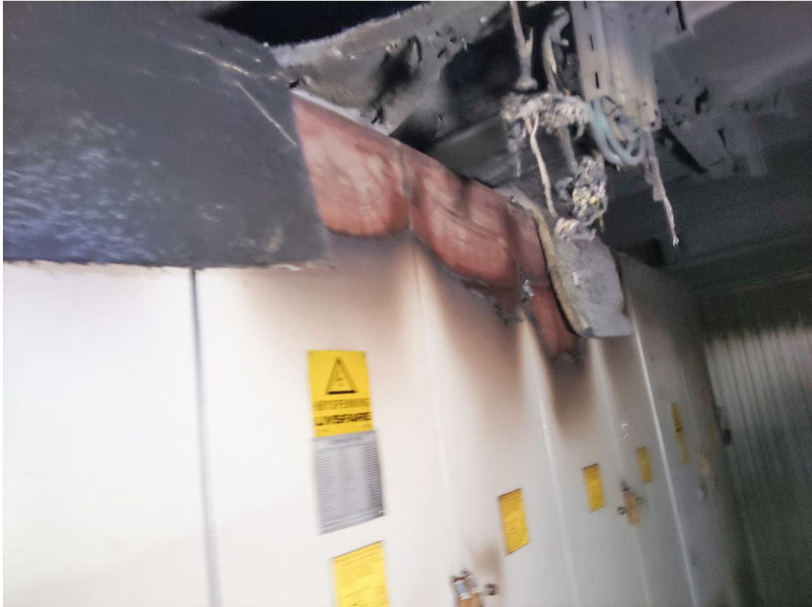
Figure 24 Thermal insulation in the ceiling above the VSD (1 of 3) (Source: Havtil)
