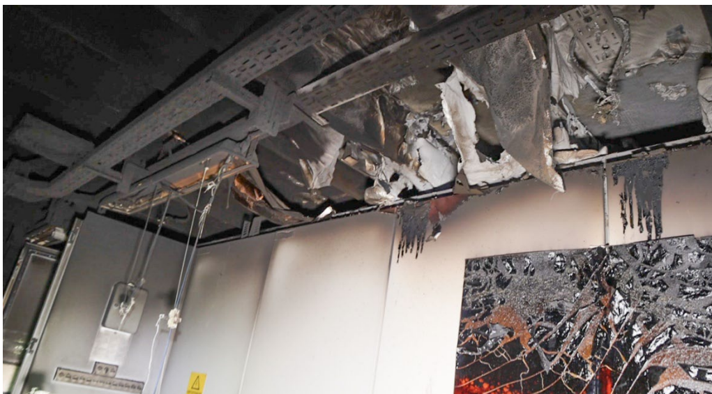
Figure 26 Thermal insulation in the ceiling above the VSD (3 of 3) (Source: Norwegian Police)
