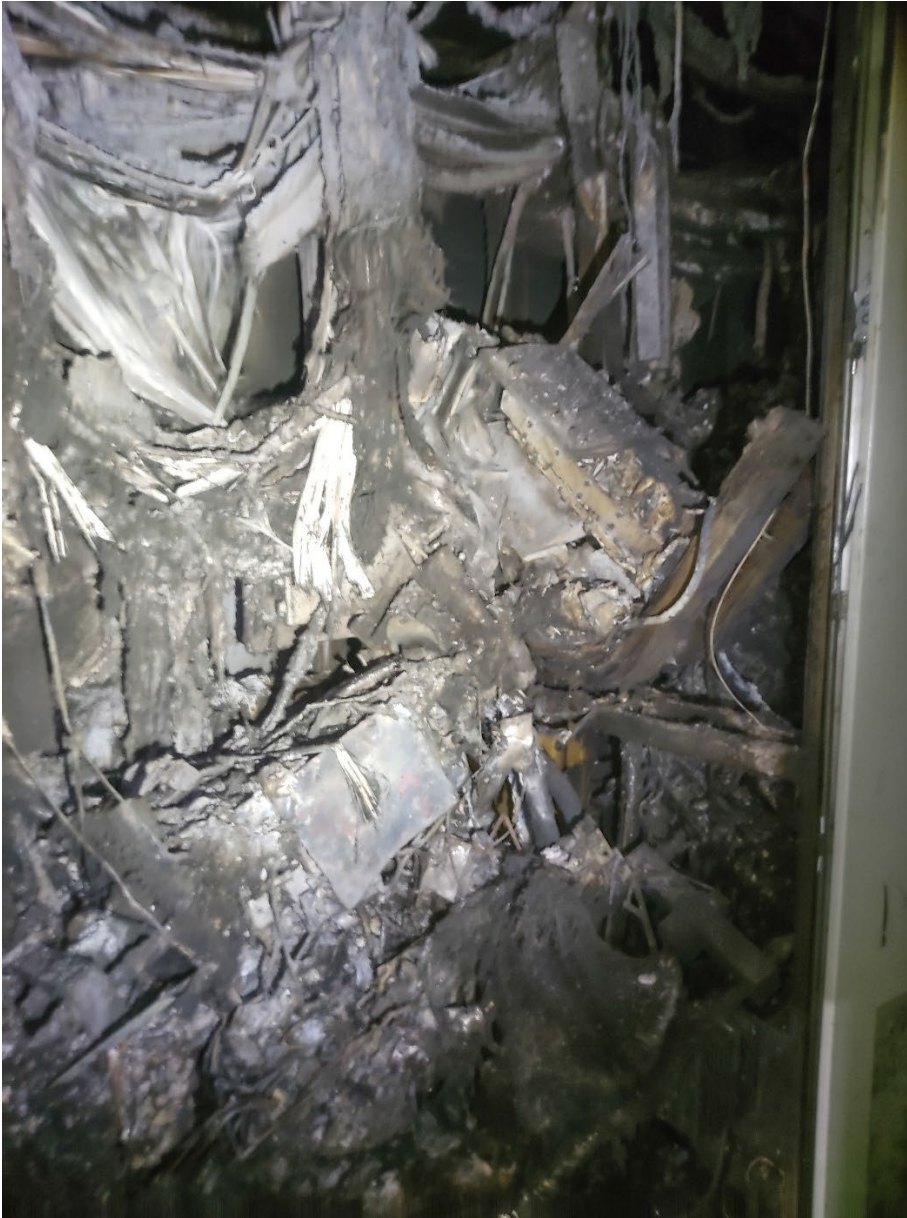
Figure 29 Fire damage to the VSD viewed from door no. 7 looking towards the output filter (Source: Norwegian Police)
