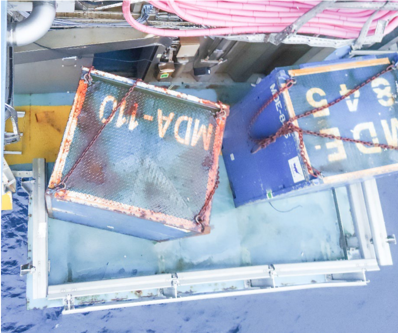
Figure 17 Pneumatic sliding door into the high voltage room. In the photograph, the two containers have been pushed towards the door as a result of being doused with water from water cannons on adjacent vessels (Source: Havtil)
