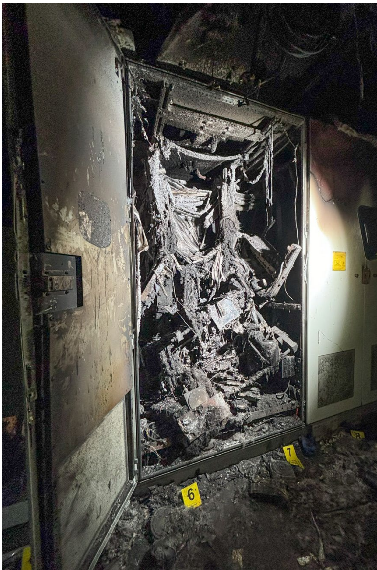
Figure 27 Fire damage to the inverter part of the VSD (Source: Norwegian Police)
