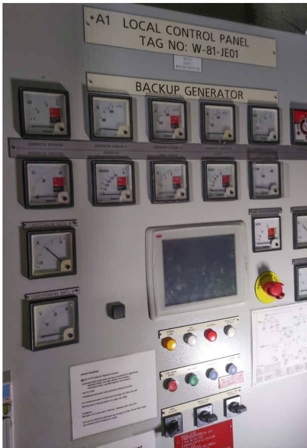
Figure 2 Local control panel for the back-up generator on SLB. The photograph was taken during Havtil's inspection after the fire. The 'Mode selector' in the bottom centre of the photograph is in Auto mode. We have unsuccessfully attempted to gain access to any alarms from the alarm panel. (Source: Havtil)
