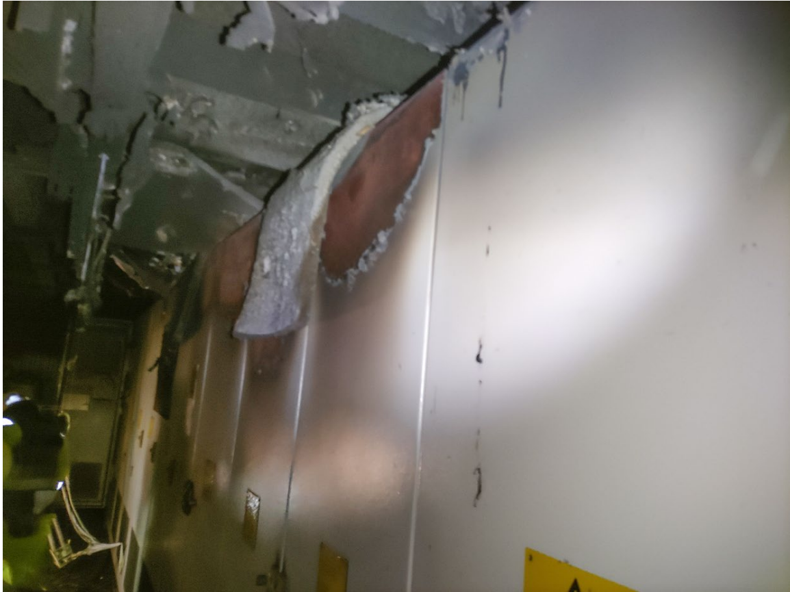
Figure 25 Thermal insulation in the ceiling above the VSD (2 of 3) (Source: Havtil)
