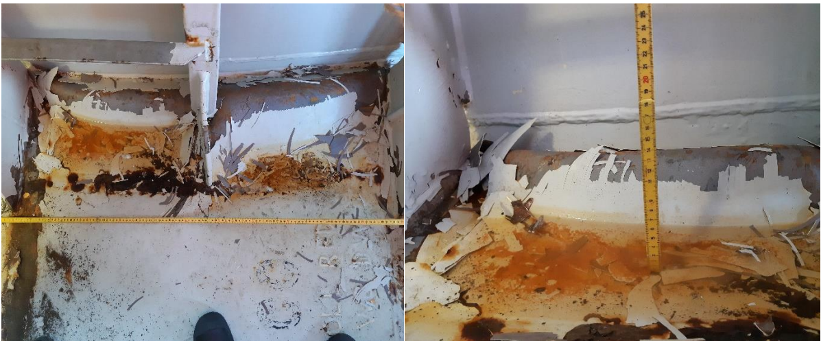
Photo: Bulged deck plate.
