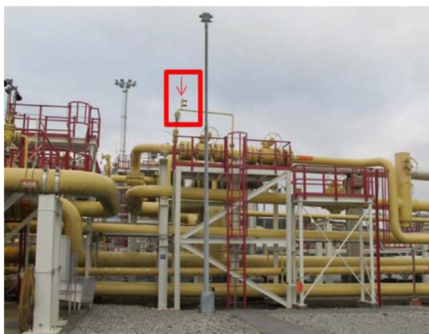
Figure 8 Photo showing the positioning of the manometer on top of a 2" bypass line seen from the south
