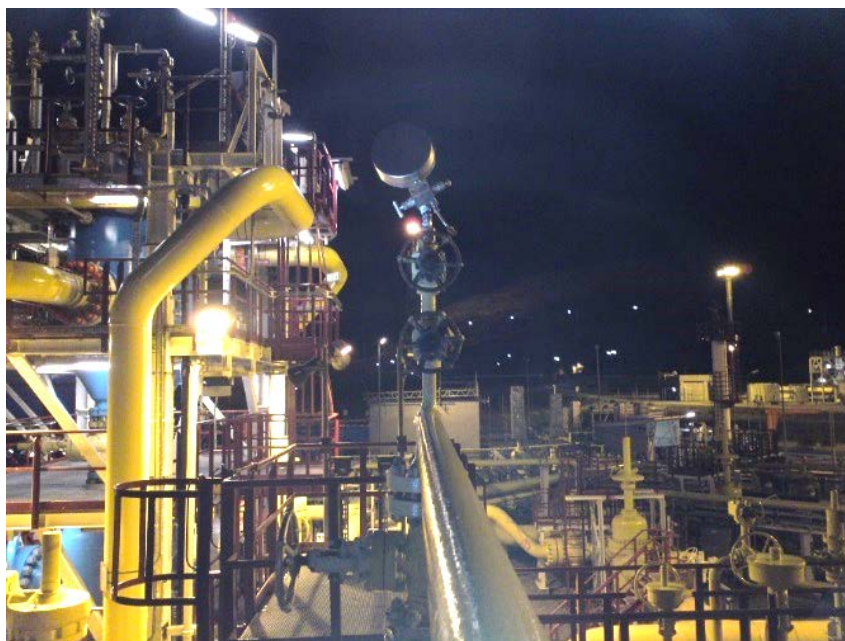
Figure 7 Photo of the manometer on top of a 2" bypass line seen from the east
