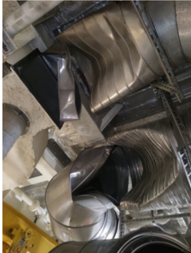
Photo 12 Exhaust ducts in the shaker room that were damaged during the incident (source: Havtil)
