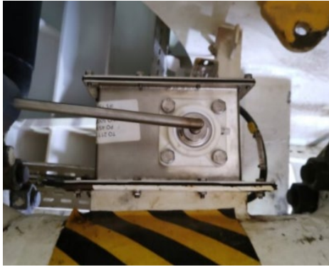
Photo 9 Flapper valve on the return flow line to the shakers (source: Havtil)
