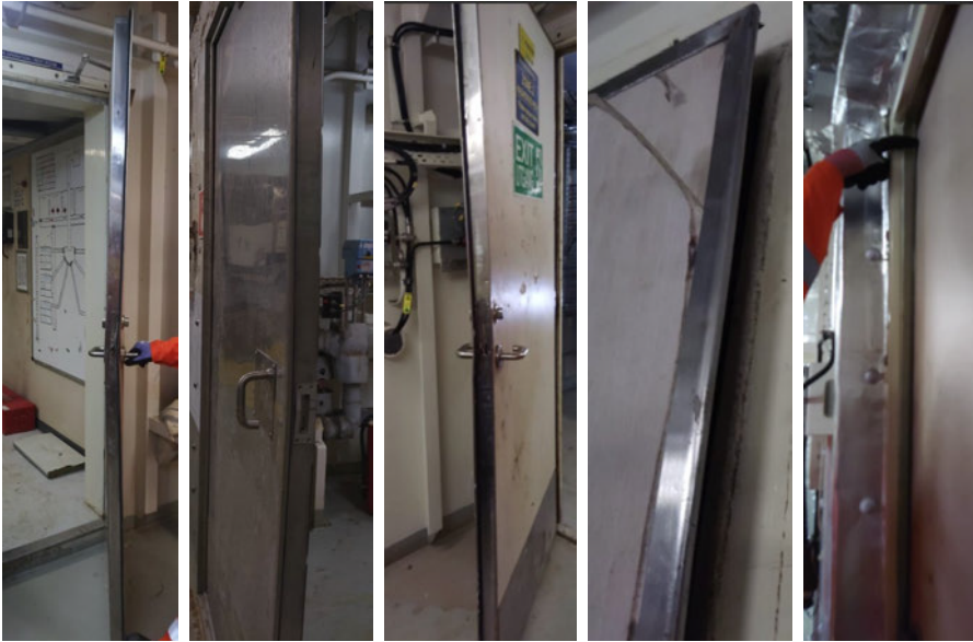
Photo 10 Examples of damage to doors in the shaker room and adjacent areas where door panels are warped or dented (source: Havtil)
