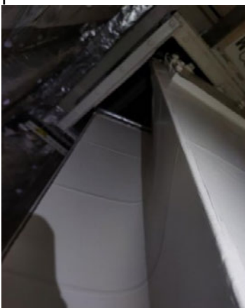
Photo 13 Imploded exhaust duct from the Shale Shaker House & Lower Part Shale Shaker located in HVAC 1 (source: Havtil)
