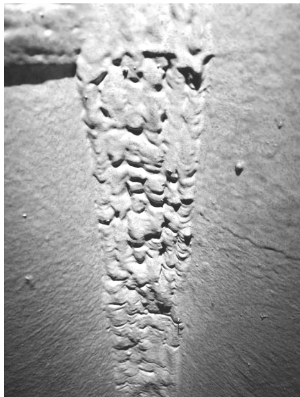
Figure 3-8 Example of poor weld quality.
