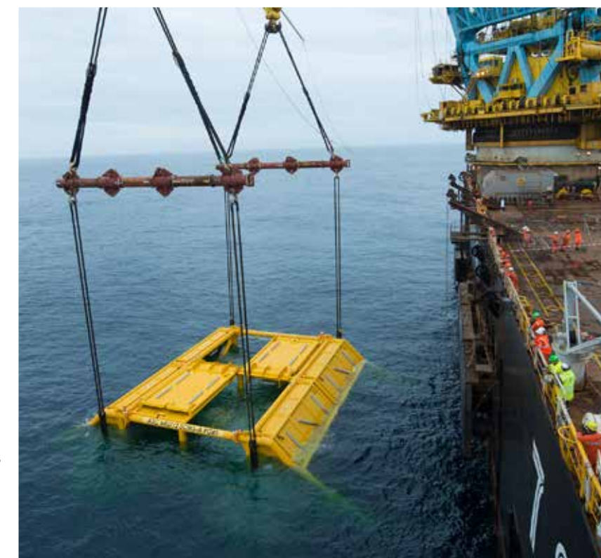
Installation work on Åsgard in the Norwegian Sea. Such subsea developments shot ahead in the 1990s. (Photo: Equinor/Øyvind Hagen)
