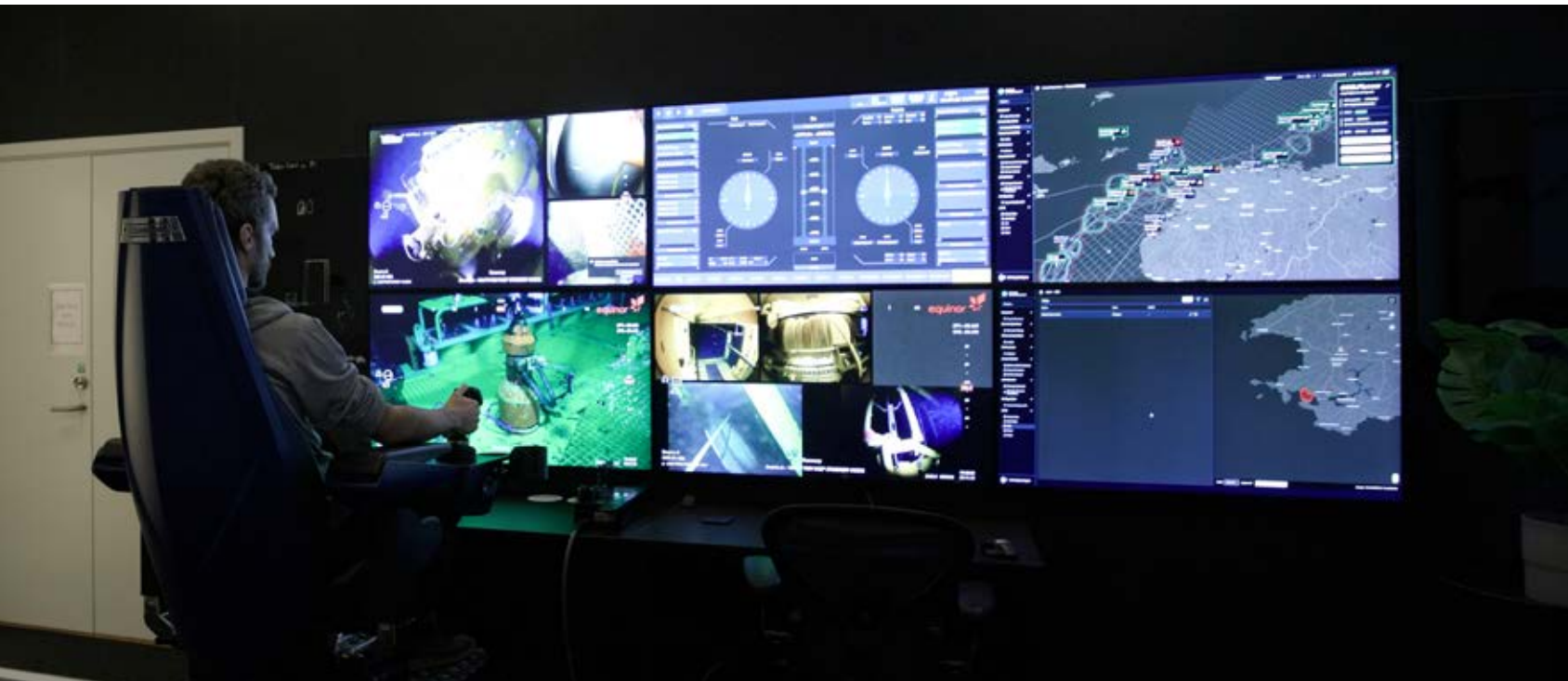
OROC is the control room from which Oceaneering controls subsea operations on the shelf and internationally – directly from land.
