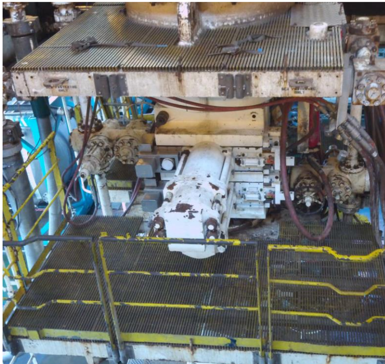
Figure 7 Access platform for the NXT BOP. Source: Valaris
