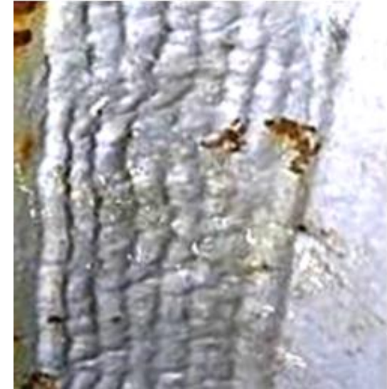
Chord to rack weld Several years in operation Grinded + MPT
