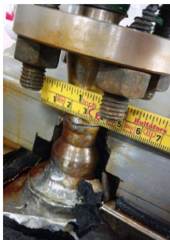
Figure 3- Crack in pipe weld which led to a condensate leak. The photograph belongs to Engie E&P
