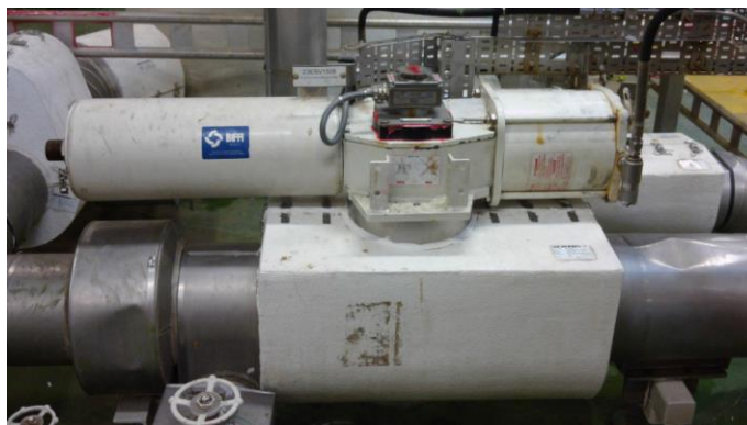
Figure 13 - ESV with installed actuator 23ESV1509, which failed during the incident. The photograph belongs to Engie E&P
