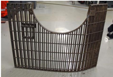
Photograph 16 Damaged deck grating plate.
