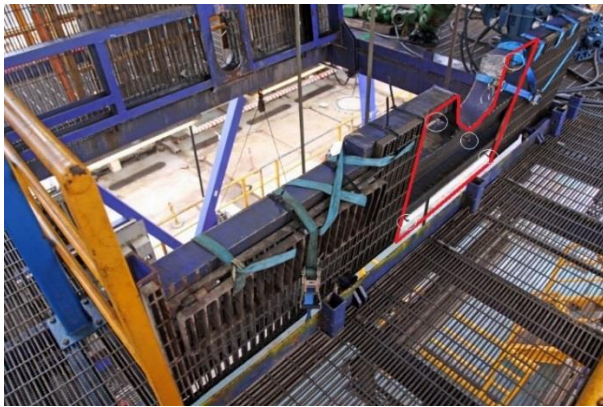
Photograph 17 Position of the grating which fell.
