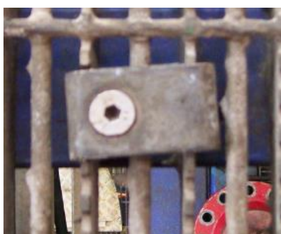
Photograph 8 Deck grating fastener.
