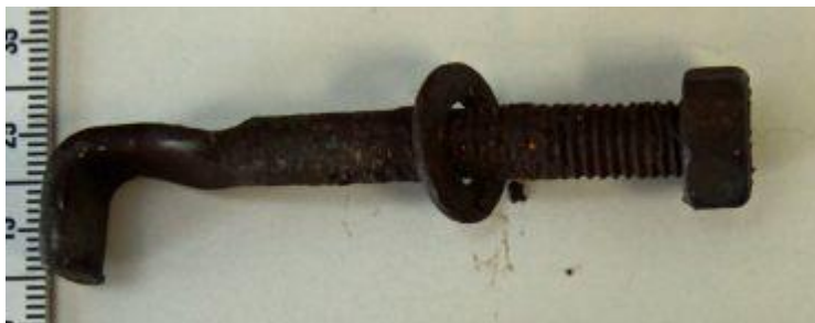
Photograph 10 Deformed J hook for the deck grating, with bolt and spring washer disassembled from the hatch where the deck grating came loose.
