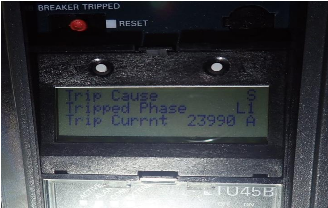
Figure 12 Trip status for incomer circuit breaker.
