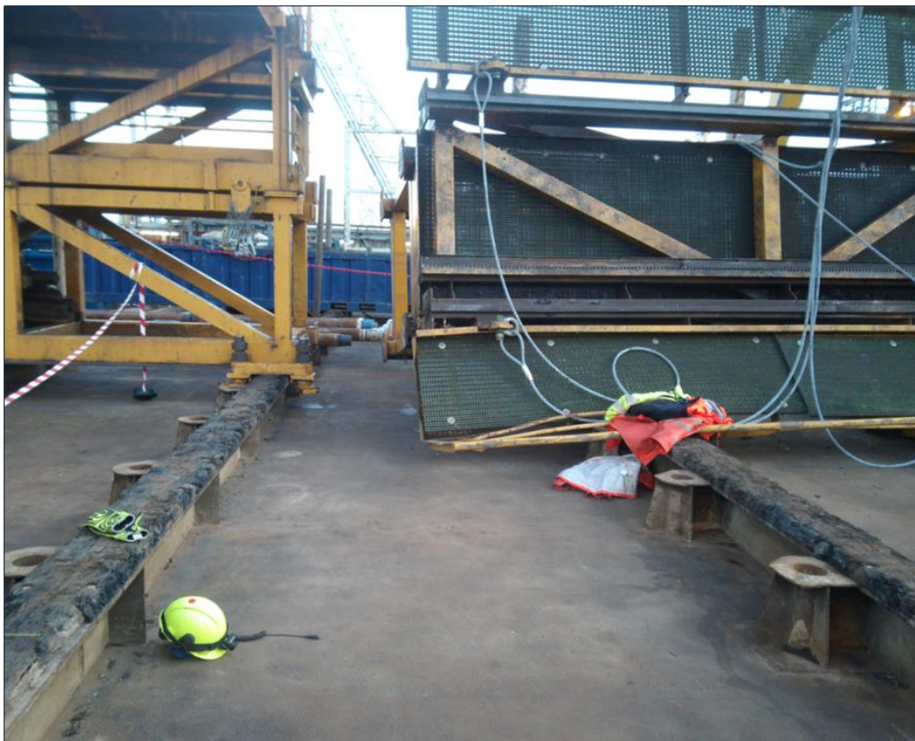
Figure 6 - The structure displaced in the longitudinal direction away from the permanent catwalk and twisted somewhat in the same direction. From Equinor's presentation of the incident.
