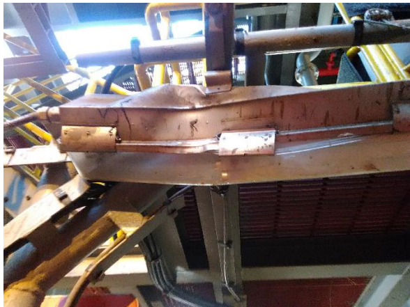
Fig 12: Damaged light fitting in the setback area.
