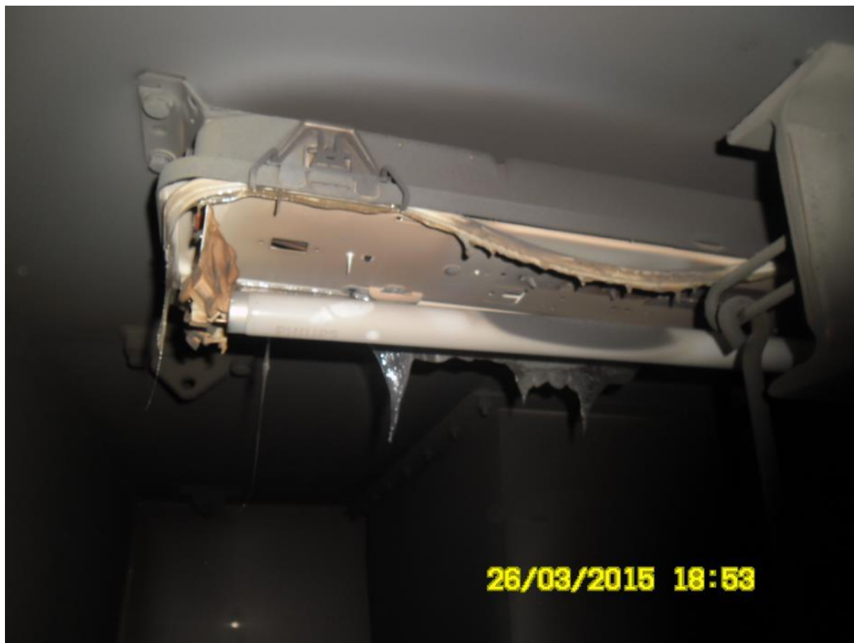
Figure 6 - Picture of light fitting in the fan housing in AHU-A (Source: PSA investigation)
