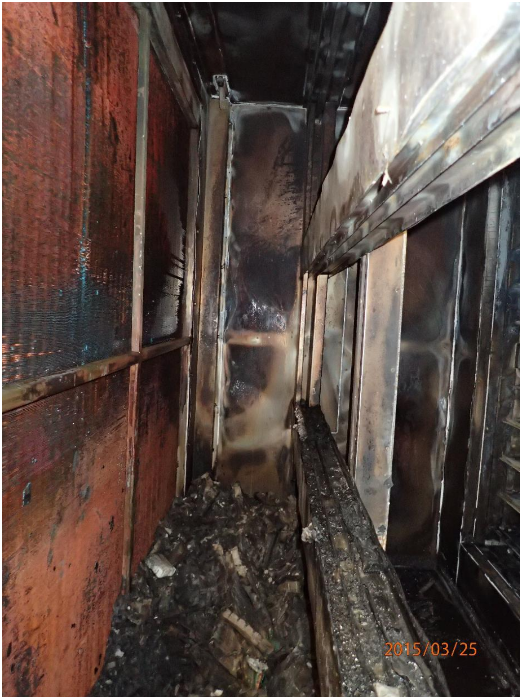
Figure 4 - Burnt-out filter cassettes in AHU-A. (Source: PSA investigation)
