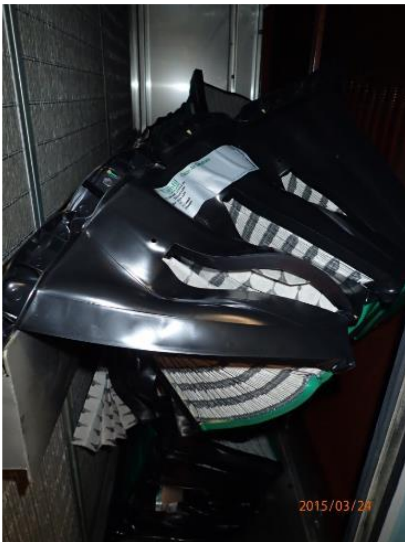
Figure 5 - Deformed cassettes in AHU-B, which is immediately adjacent to AHU-A (Source: PSA investigation).
