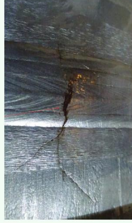
Pic. 2: Field observation on gas cooler.
