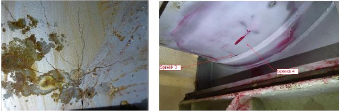
Figure 9: Visual images of crack 1 (left) and penetrant indications of cracks 3 and 4 (right). (Photos: Equinor)
