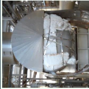
Pic. 1: Gas cooler after partly removal of insulation.
