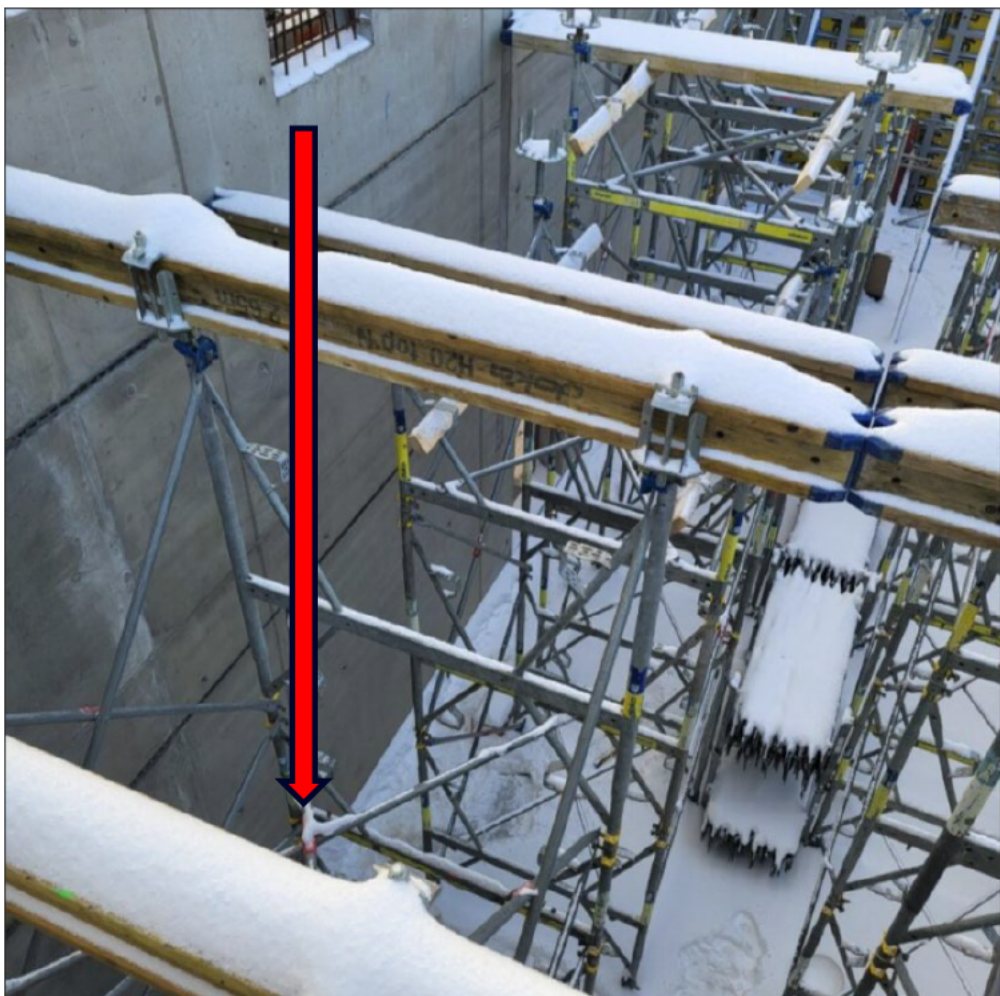
Figure 1 The formwork scaffolding where the fall accident occurred on 24 April 2025
