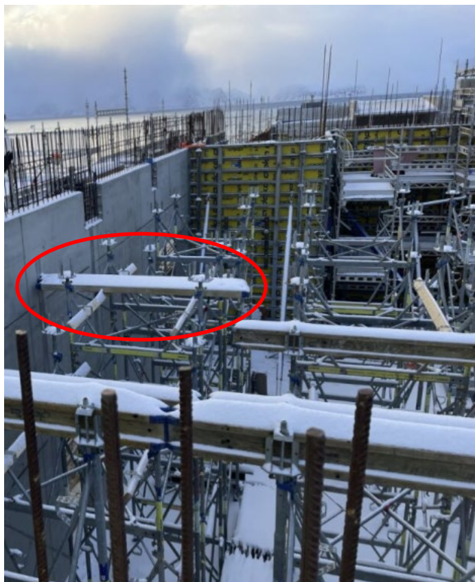
Figure 3 The image shows how Doka beams were laid as a base in the absence of Doka flooring. The red circle clearly shows how the beams protrude beyond the support beam on which they rest.
