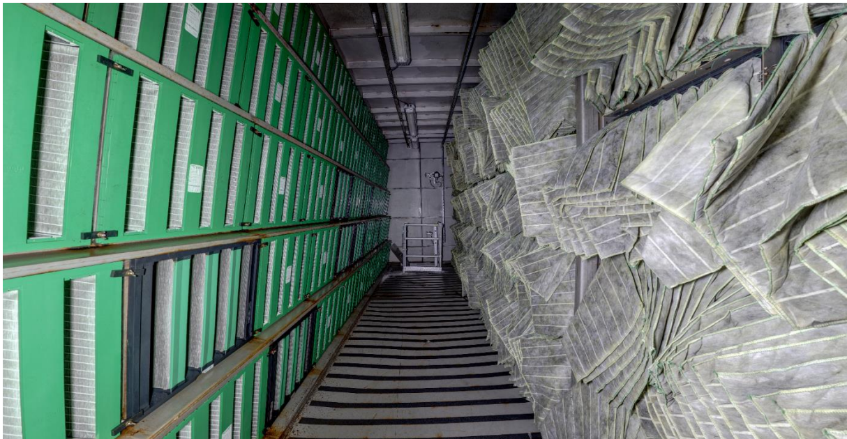
Illustration 4 GTG5 filter housing, second level. Pre-filters right and fine filters left (Photo: Kripas)
