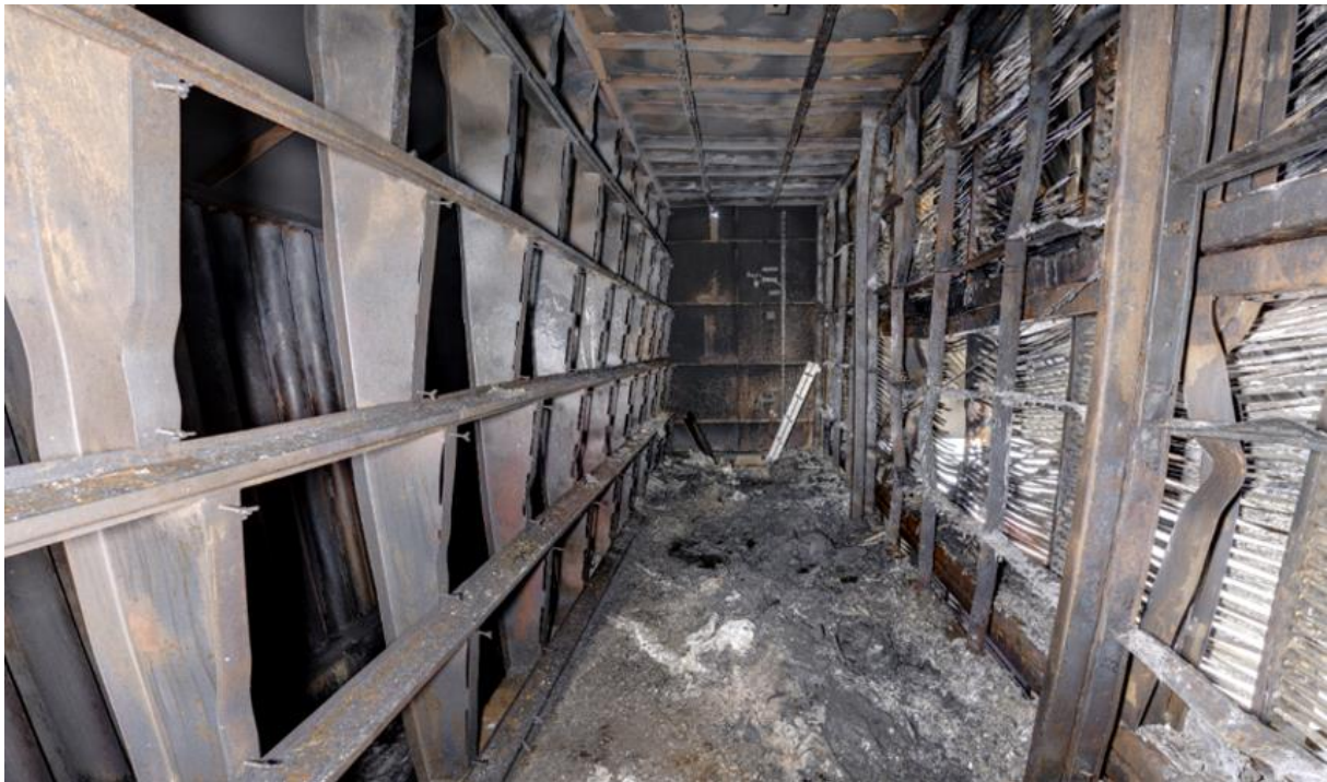
Illustration 10 Interior of the GTG4 filter housing, level 2, after the fire (Photo: Kripos)
