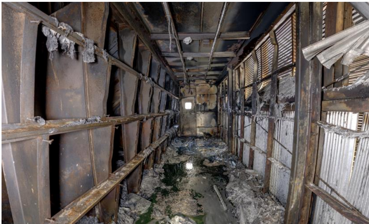
Illustration 9 Interior of the GTG4 filter housing, level 1, after the fire (Photo: Kripas)
