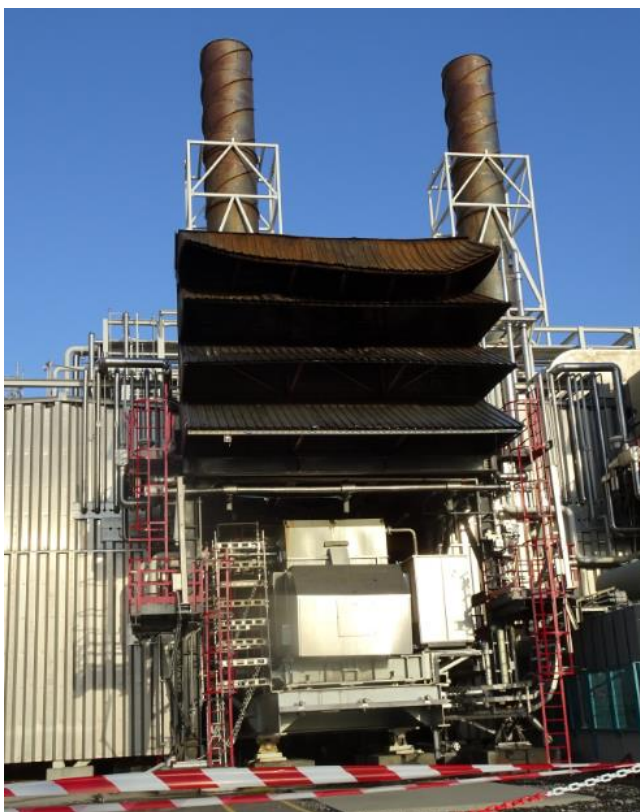
Illustration 11 External view of the damage to the GTG4 air intake (Photo: PSA/AHS)
