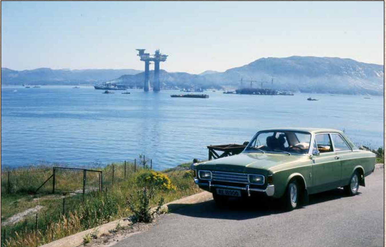
Platforms under construction in the Gands Fjord off Stavanger in the mid-1970s. Norway's oil history is not only about big structures and engineering skills, but also about the creation of a safety regime – about regulations and accidents, audits and triumphs, the Norwegian model, and trust and responsibility. The Norwegian Petroleum Directorate, and later the PSA, have played a key role in shaping the system which underpins today's level of safety. (Photo: Øivind Anda Pettersen/Norwegian Petroleum Museum)
