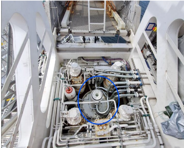
Photo 5: Swivel and hydraulic pipe spools (Source: Equinor/Island Offshore)
