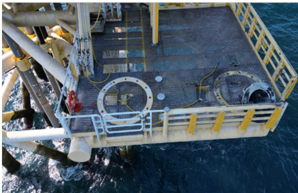
Photo 6: Landing platform with damaged deck grating and Equinor/Island Offshore) detached cone (Source: Equinor/Island Offshore)
