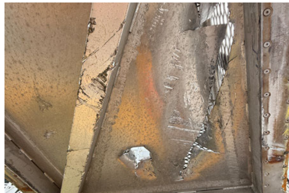
Photo 7: Damage to the gangway (Source: Equinor/Island Offshore)
