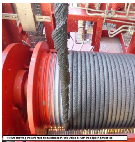
Figure 3 Damage to the steel rope on the HTV Eagle crane. (Synergi # 1461090, January 2016)
