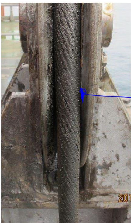
Figure 5: The steel rope bearing against the sheave.
