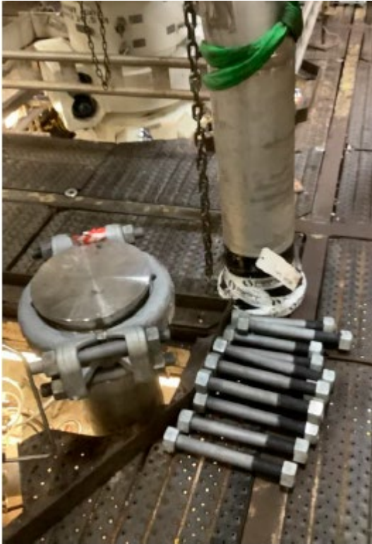
Figure 9 Photograph of the incident site. It was taken before work on splitting the blind hub began on the day of the incident. (Source: Equinor)
