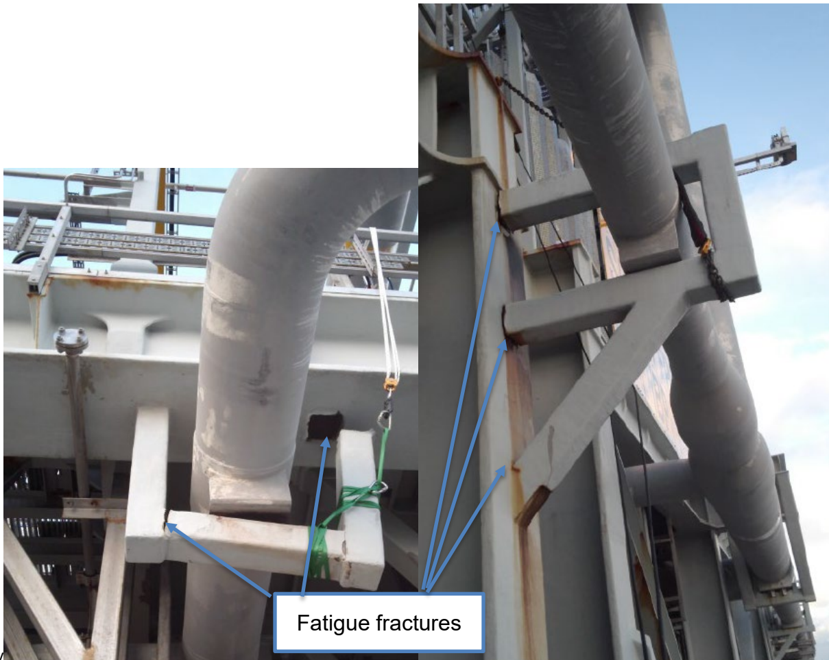
Figure 3-9 Example of two adjacent, welded pipe supports (RHS 150 and RHS200) failed by fatigue. Photos used with permission from operator.
